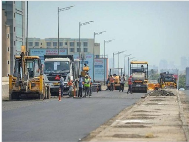
Earthmovers are seen on Andheri flyover to complete the repair work as instructed by the state government during a nationwide lockdown in the wake of coronavirus pandemic, in Mumbai. Photo: PTI
