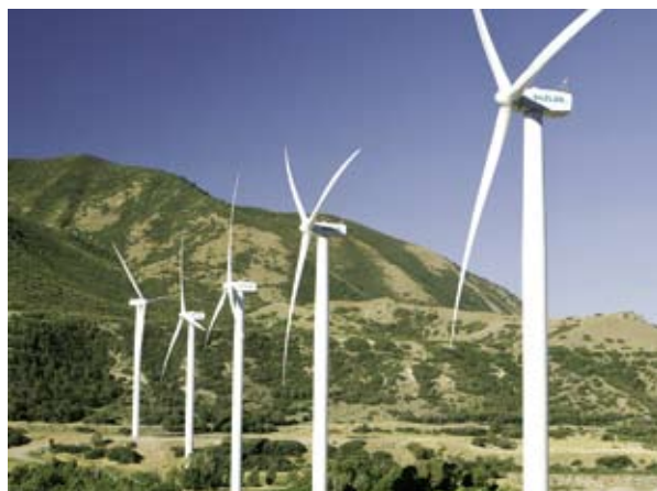
Suzlon wind turbines, Spanish Fork
